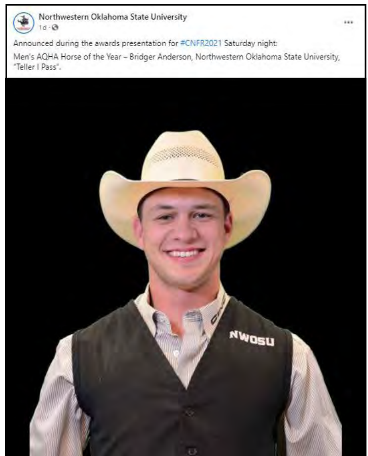
Work continues in Ryerson Hall on the final two restroom renovations. Left and top left are first floor restrooms. This area will now house a women’s restroom and private restroom. Second floor renovation is for a women’s restroom.
