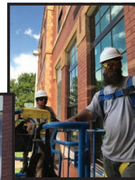
We've had campus staff (left) and contractors (above) involved with the window update.
